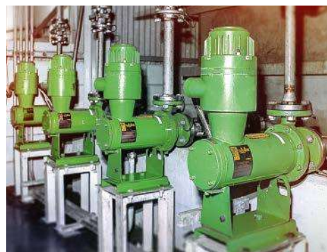
Basic type pumps in a chemical plant.
